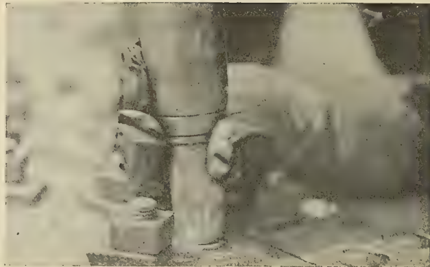
Fig. 14.—Riveting Between Service Bolts With Proposed Standard Set, Showing Ease With Which Set is Used. Rivet Being Driven Straight Down to Swell the Shank of Rivet and Fill Hole
